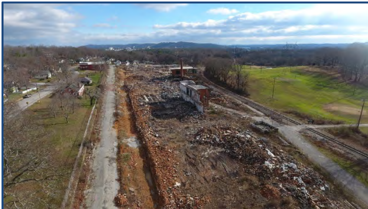
Before the former Lupton City Mill site was cleaned up, hazardous debris, including asbestos, was spread across the 12-acre property.
