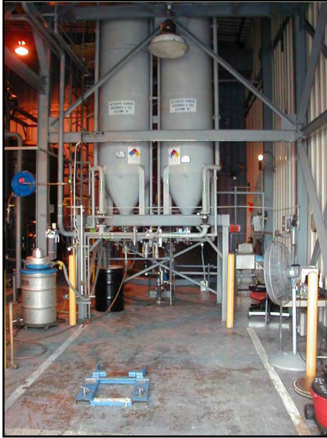
Fig. A.3. GWTF located in Bldg. 9616-7.
