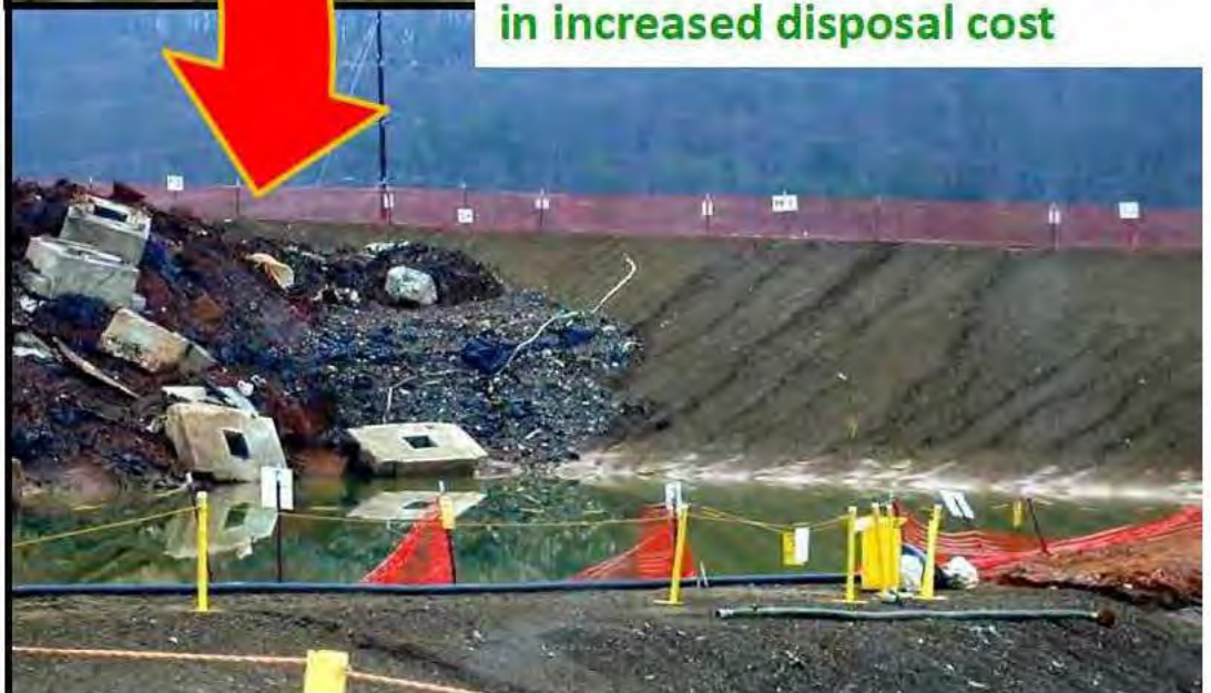
Demolition and remediation waste landfilled in 2002 at the Environmental Management Waste Management Facility (EMWMF)
