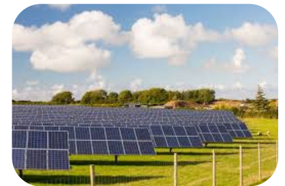
Renewable Energy Generation
