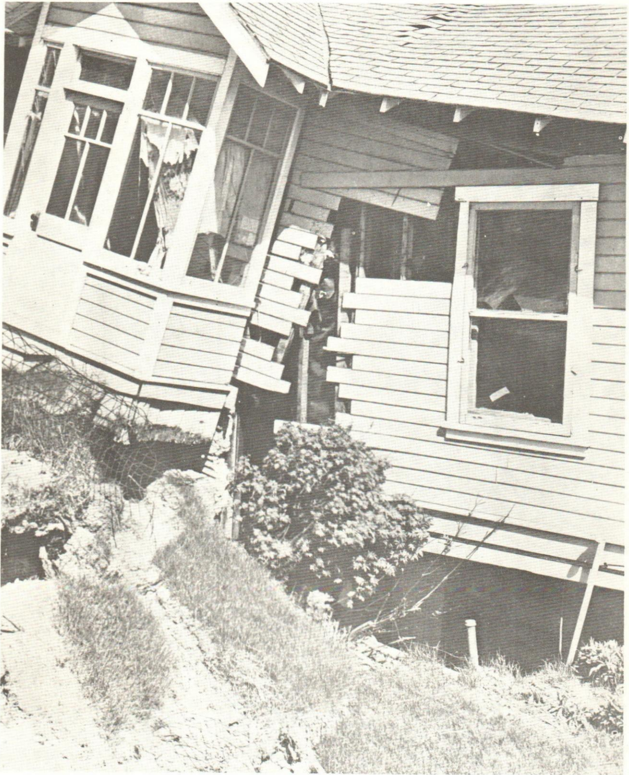
Figure 10C. Wreckage of a dwelling that was partly on collapsed ground. Such damage is likely from a violent earthquake in Tennessee. Reprinted from U.S. Geological Survey Professional Paper 542A, p. A46.
