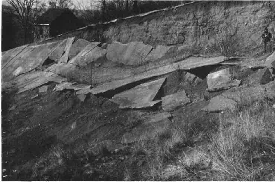
Figure 19. In an unsuccessful effort to stabilize the slopes at EMIN 8, a layer of gunite was applied. This resulted in the large, broken slabs visible in the photograph.
