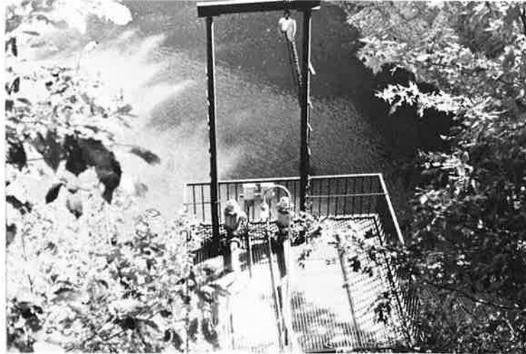
Figure 2. Twin pumps lift water for use by Mowbray Mountain Utility District.
