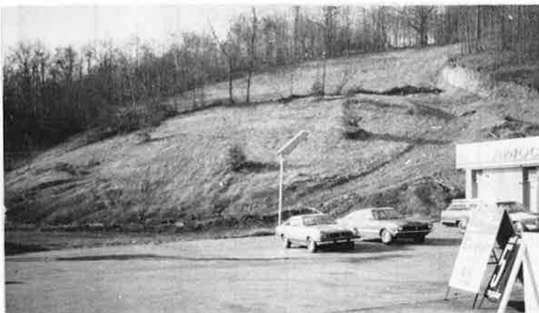
Figure 14. Part of the landslide located at EMIN 10 that has been abutted by the back of a business establishment.
