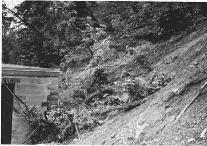
Figure 15. Small landslide in Knox Group colluvium and residuum located at EMIN 18 (Lakeshore Drive).
