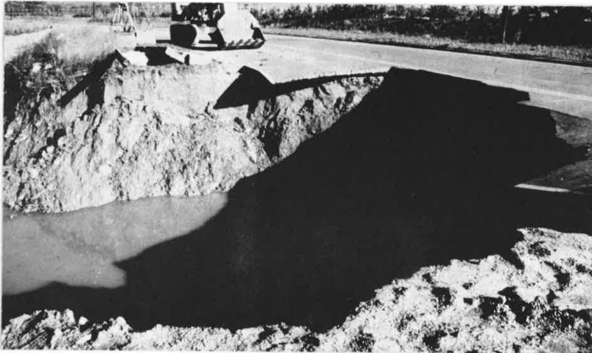
Figure 21. Sinkhole in Airport Road approximately 2 miles (3.2km) north of northernmost extension of the Chattanooga Municipal Airport.
