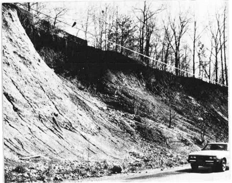
Figure 13. Landslide scarp in Knox Group residuum and colluvium located at EMIN 10 (junction of Tenn. Hwy. 58 and Tunnel Blvd.). Soil benching has been utilized in an attempt to stabilize the slope.
