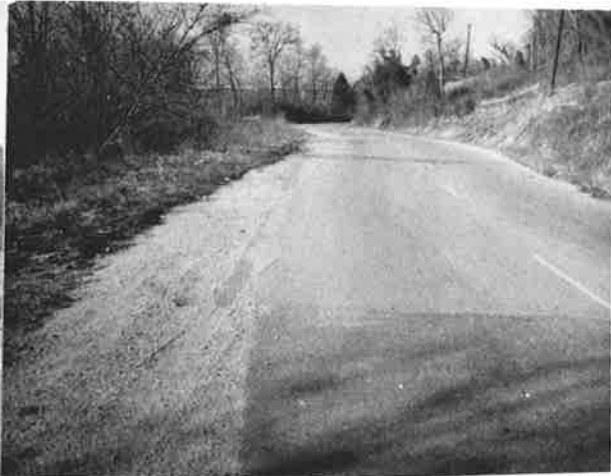
Figure 17. The landslide at EMIN 11 (note tilted tree in upper left part of photograph) resulted in a new roadway alignment. The road shoulder of Lakeshore Drive, which was realigned, originally followed the white, dashed line.
