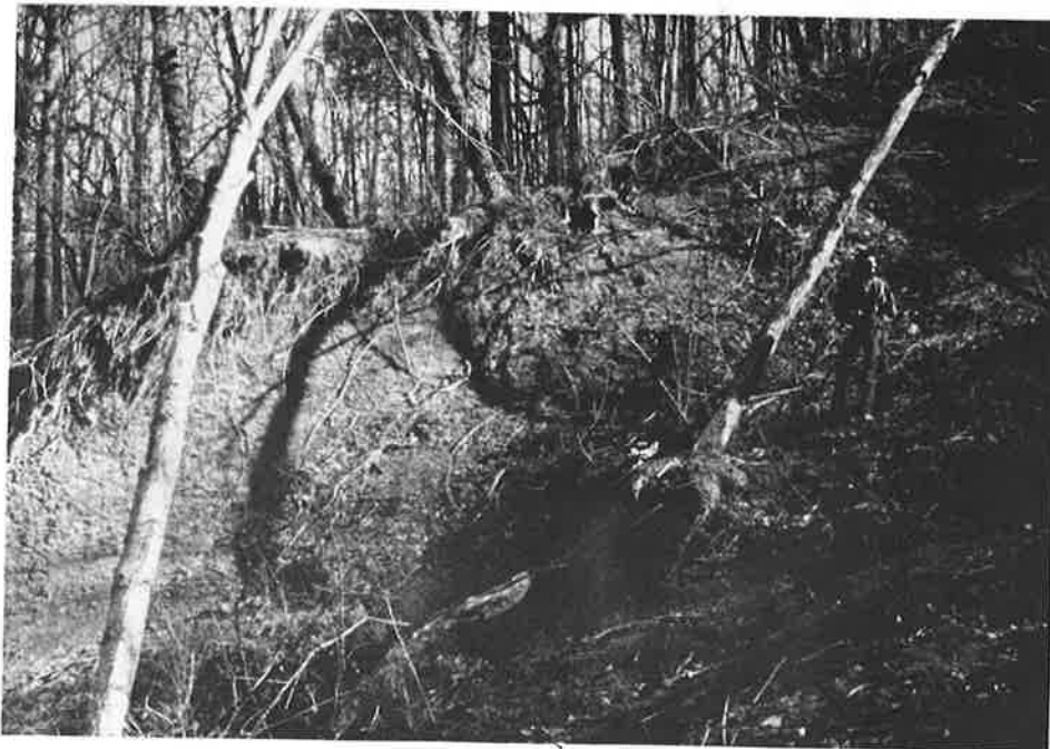
Figure 5. Toe area of Pennington landslide located at EMIN 1.
