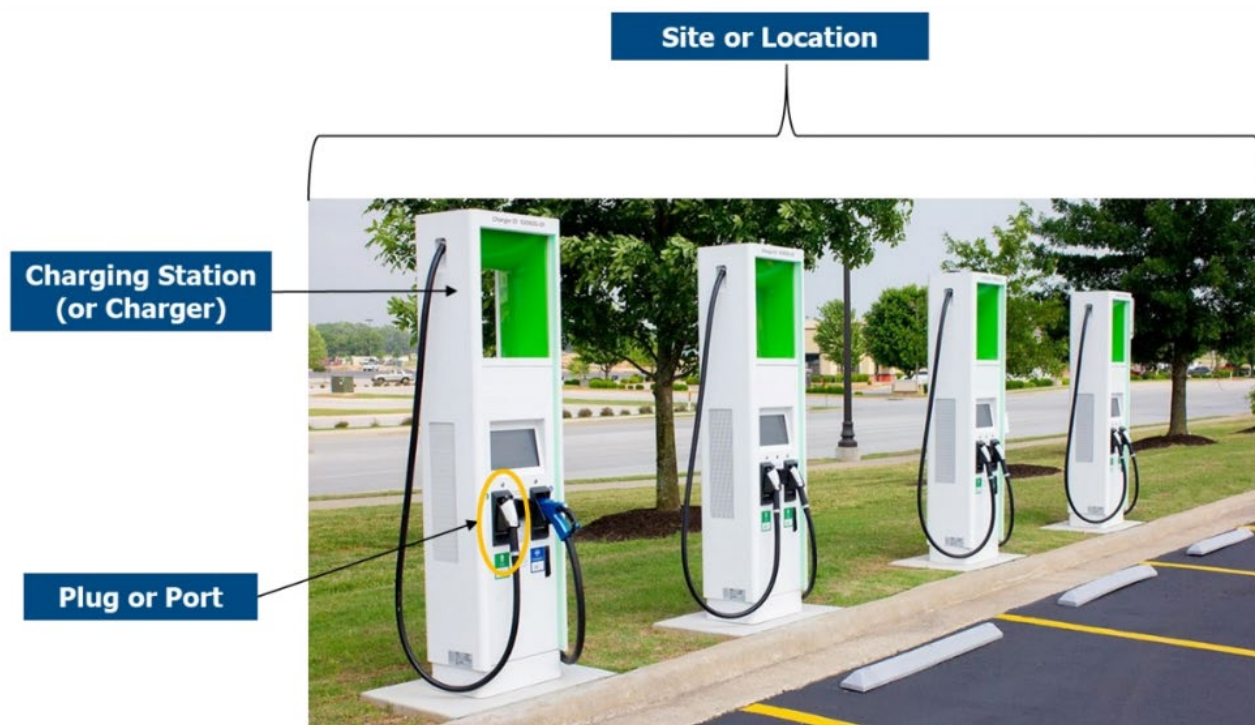
Figure 1. Example Fast Charging Site and Terminology
