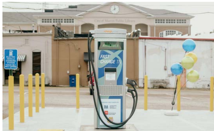
Fast Charge TN Network charger installed in Martin.
