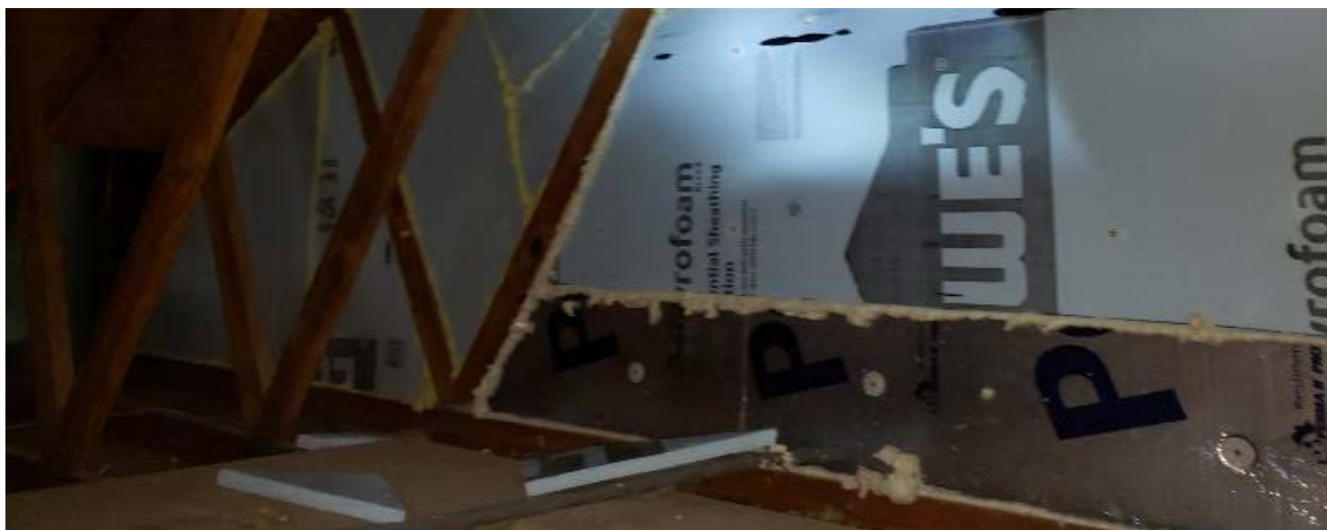
Home Uplift home's attic before, with no insulation.
