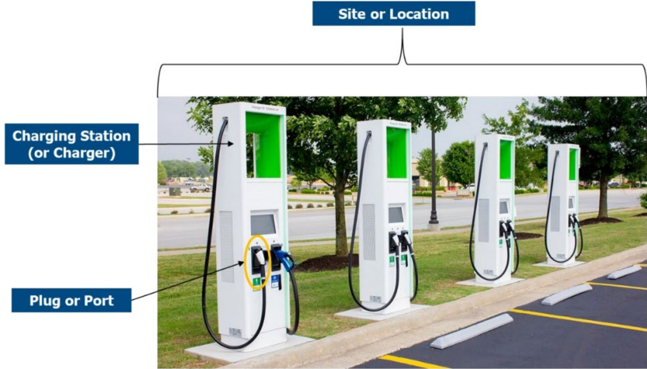
Figure 1. Example Fast Charging Site and Terminology
