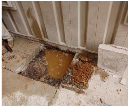
Figure 6.3.1a – Department of Military Water Leak
