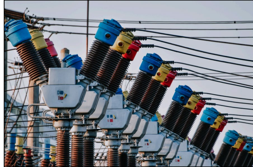
Electricity poles and transformers by Diana
