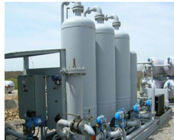
Natural Gas Compressors
