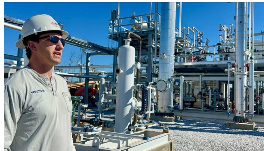
Natural Gas Processing
