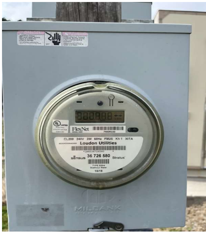
Photo: 012 Date: 02/25/26 Photographer: EMH Description: Electric meter
