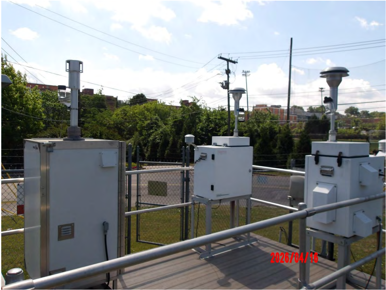
Figure 30: Sampler/monitor inlets at the Siskin site
