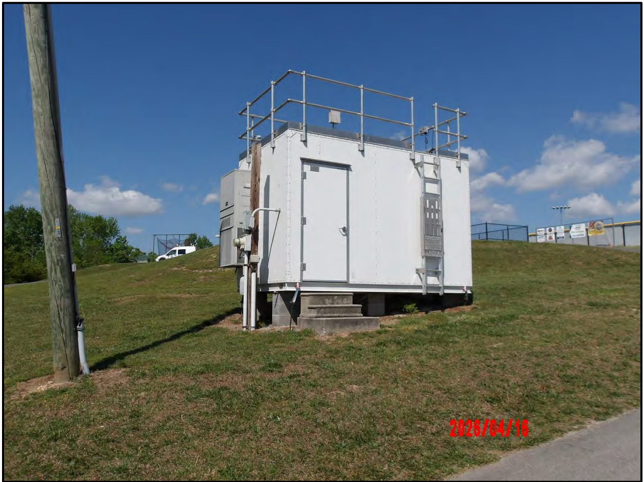
Figure 23: Current ozone monitor shelter at Soddy Daisy
