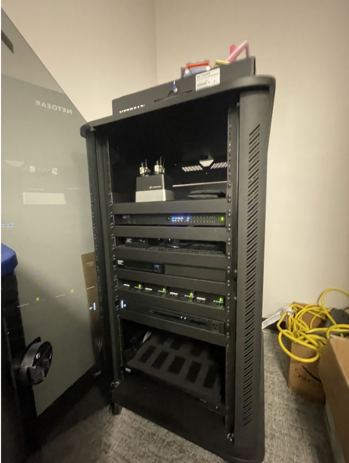
Photo 4: Network Switches in a Connected Community Facility in Davidson County, Tennessee
