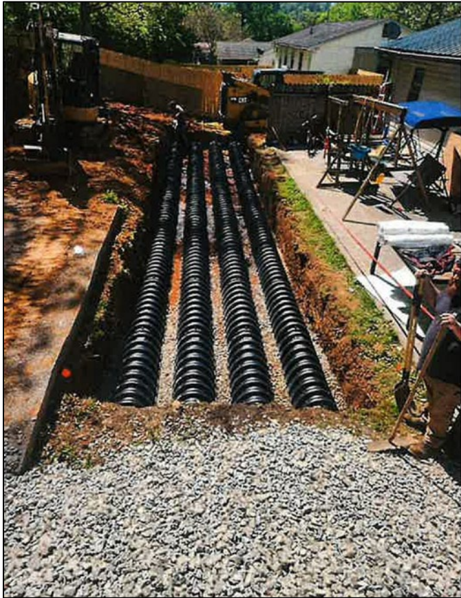
Photograph 1: 2-foot chambered septic field line
