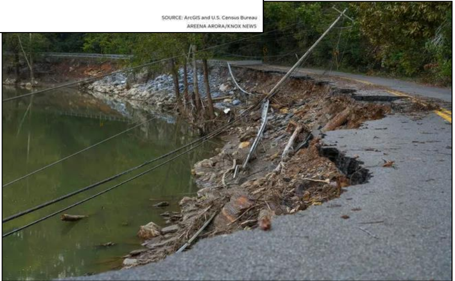
Right: Infrastructure damage from Hurricane Helene in Carter County
