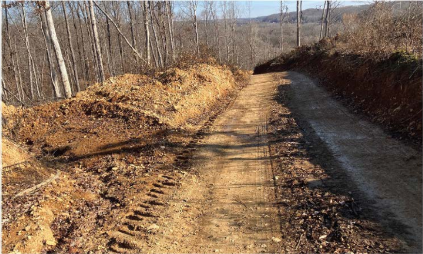
Figure 3. Main log road with turn out.
