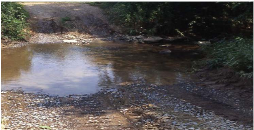
Figure 8b. Correctly Constructed Ford
