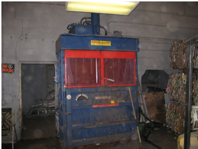
Vertical Baler at Recycling Facility
