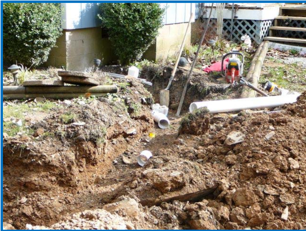
Plumbing from residence to new septic tank
